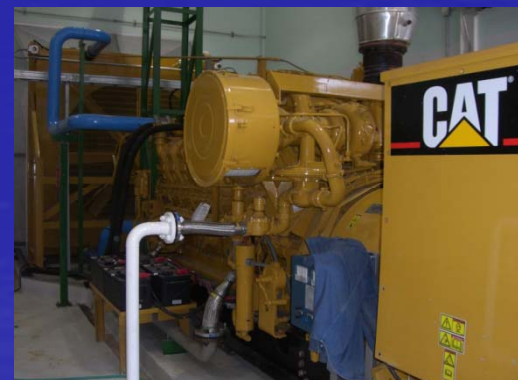
Electricity for Small Generator
